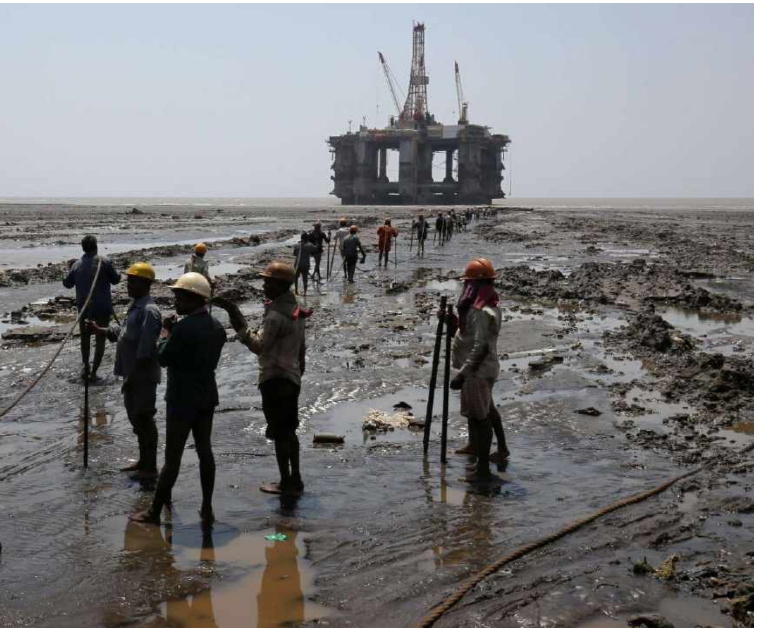
Workers prepare to tie a rope to a decommissioned oil rig to dismantle it in Alang, India © REUTERS/AMIT DAVE - 2018
