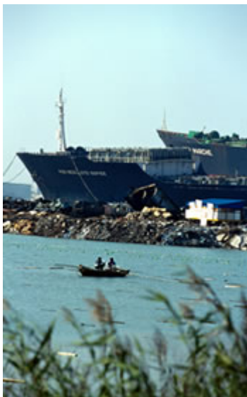
In China shipbreaking looks less dramatic than on Indian or Bangladeshi beaches. Vessels are broken up in docks with more cranes and machinery. But in fact the working conditions are similar in shipbreaking yards all over Asia
